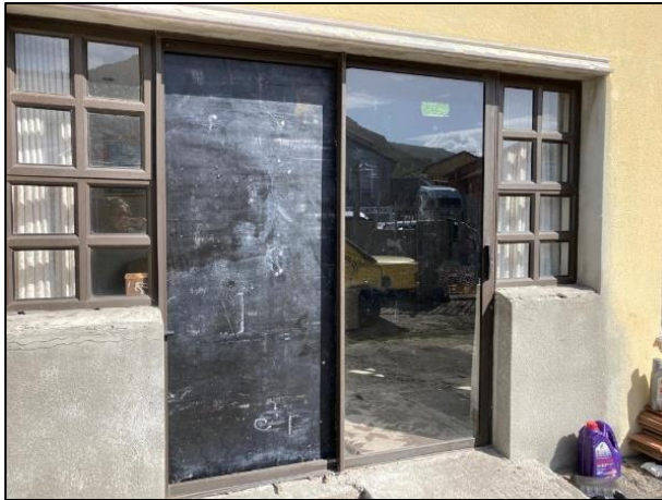
Figure 2. Baboon damage to a sliding door in Ocean View
