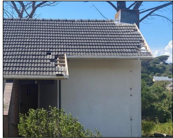
Figure 3. Baboon damage to a roof in Da Gama Park
