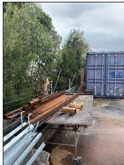
Figure 8. Vegetation and containers preventing progress on the electric fence at Heron Park.
